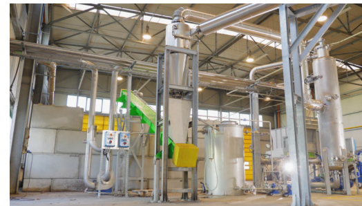
The output of the reactor passes through a cyclone to separate the solid exploded biomass from the steam, which is condensed and sprayed onto the biomass to increase the moisture content.
